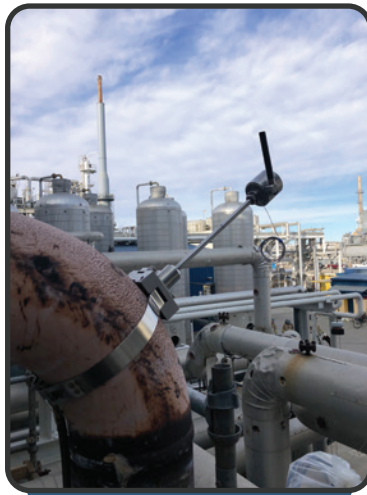
Ultra-high-temp installed using a band clamp
