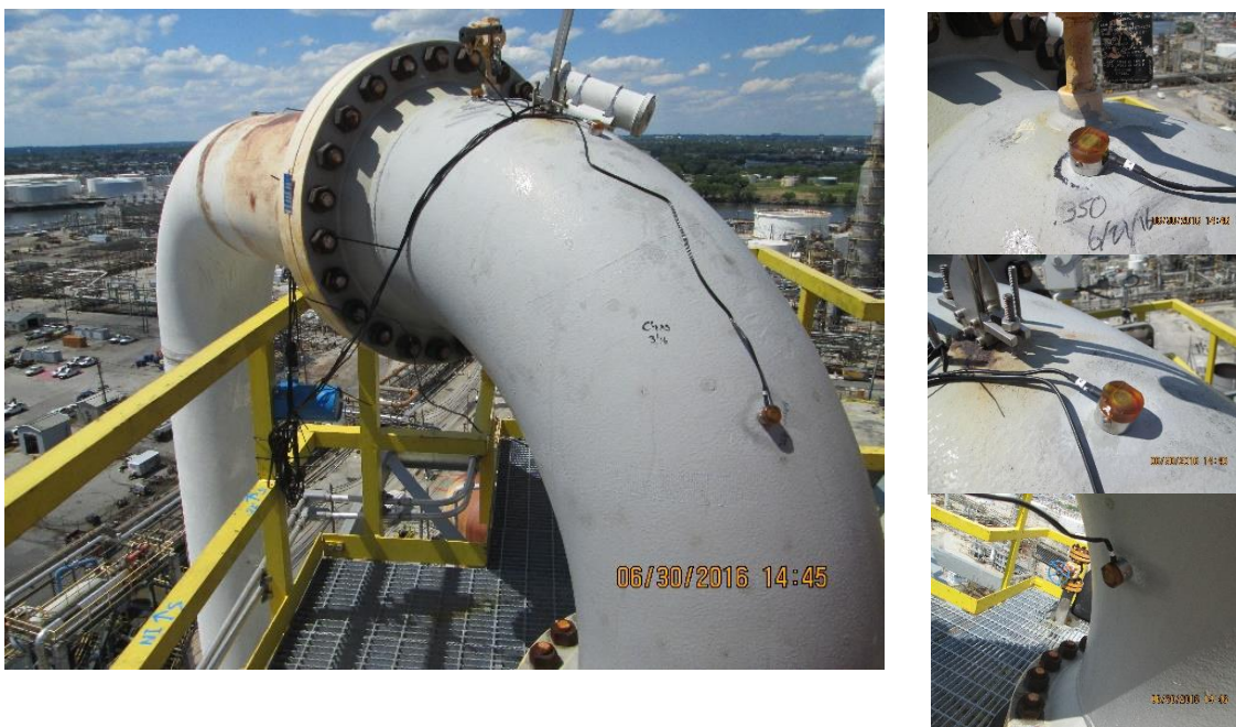
Figure 4: HF alky monitoring installation.
