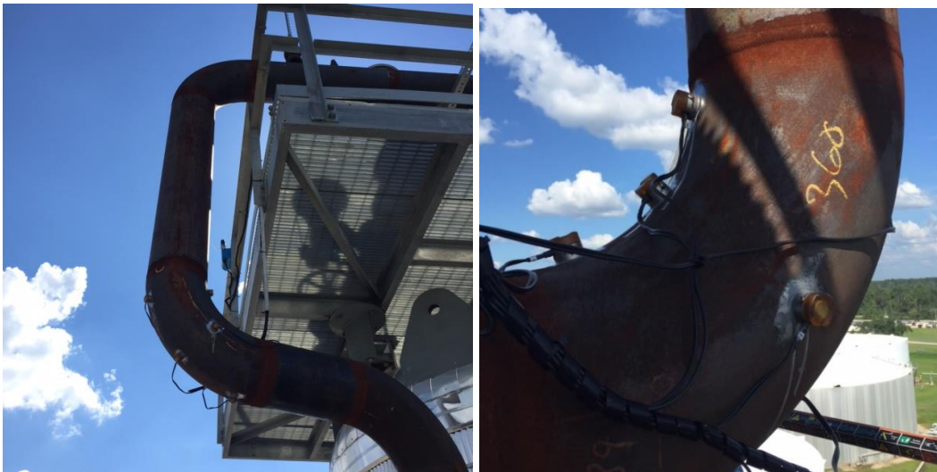
Figure 8: Sensors mounted on a crude unit overhead line.
